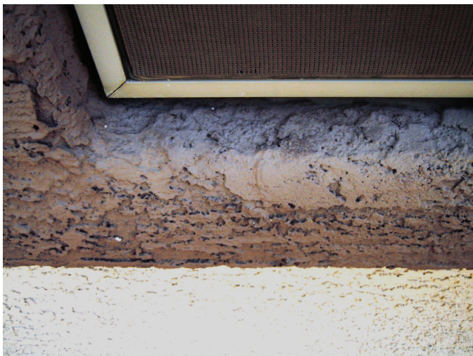
Figure 1: Premature degradation of dark colored paint on horizontal surface.
